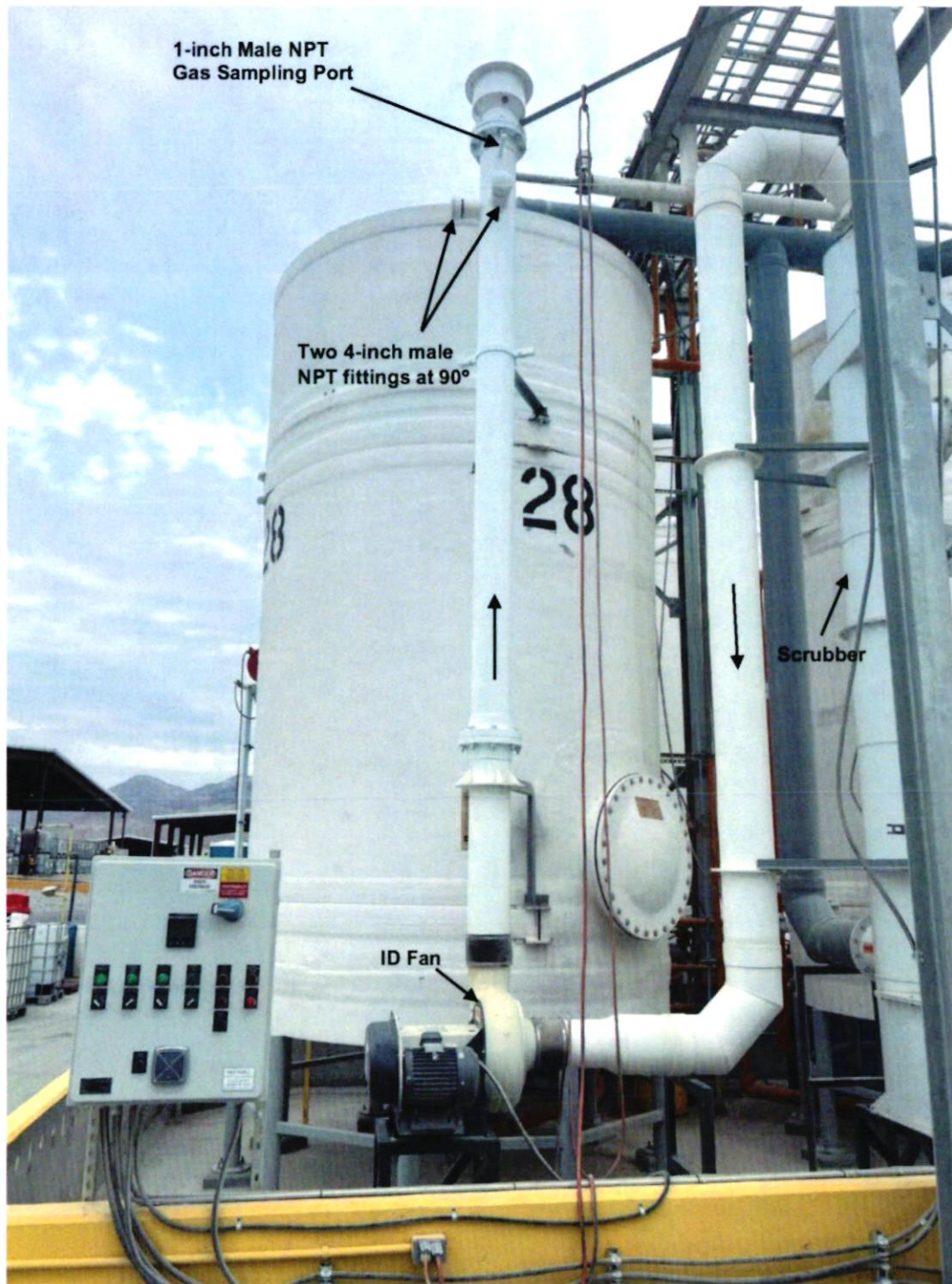
Figure 2. System 26a, Scrubber #1 Sampling Location.
